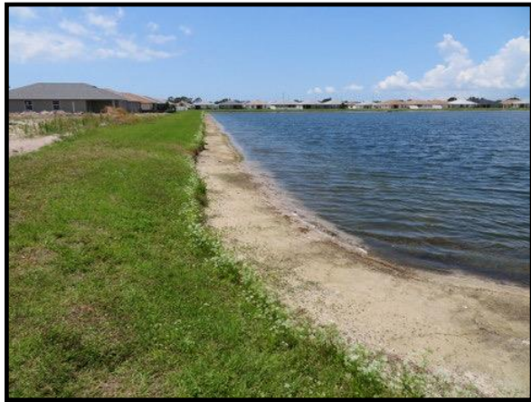
Figure 3 – Phase 5 Pond Erosion
