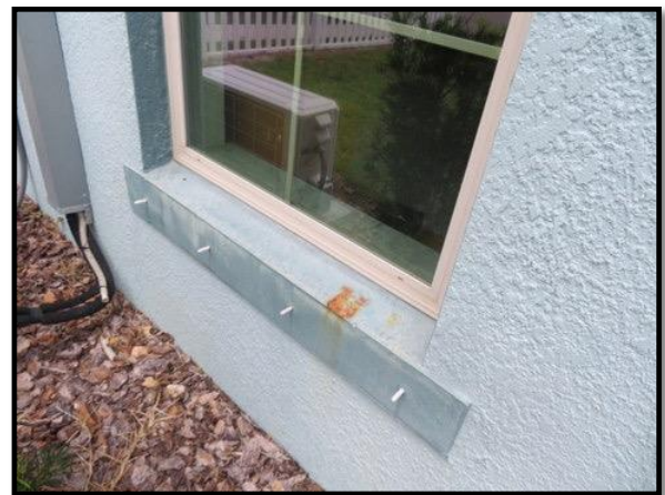
Figure 2 - Faded Paint at Maintenance Building
