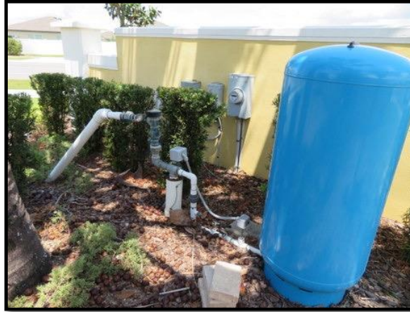
Figure 1 – Phase 4 Pump Station
