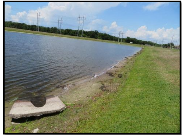
Figure 2 - Phase 2 Pond Erosion
