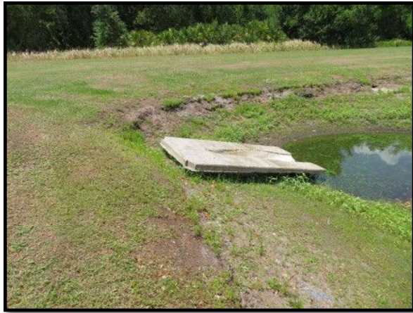
Figure 1 – Phase 1 Pond Erosion
