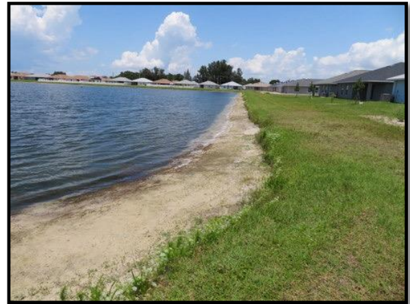
Figure 4 - Phase 5 Pond Erosion
