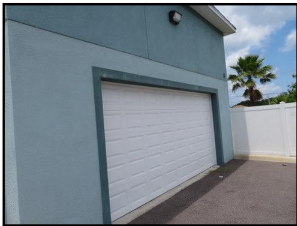
Figure 1 – Faded Paint at Maintenance Building
