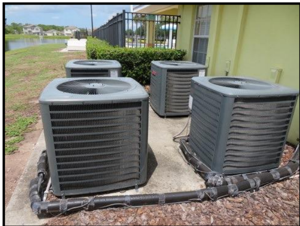
Figure 1 – Split System Condensing Units
